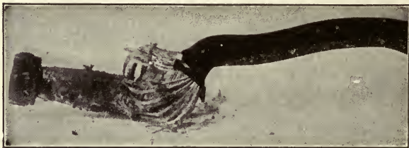
FIG. 64.—Effect of corrosion on battery cable terminals.
